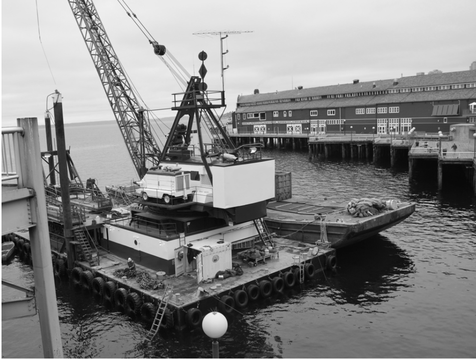
Photo 1: Crane barge at incident site (photo taken over a year later).
