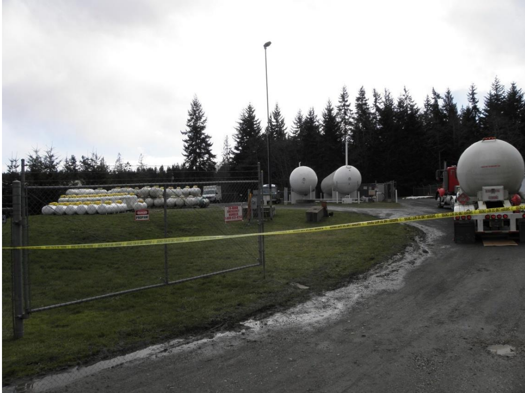
Photo 2. Propane bulk plant facility. Incident propane transport on far right.
