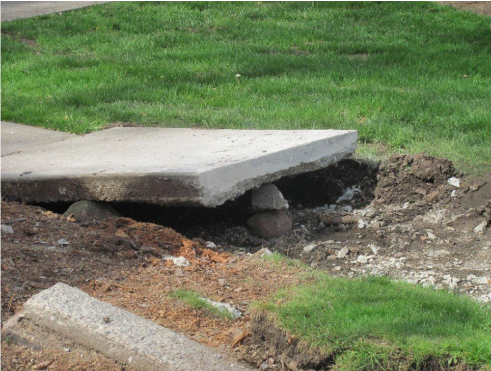
FIGURE 2: Sidewalk slab propped-up by stones.
