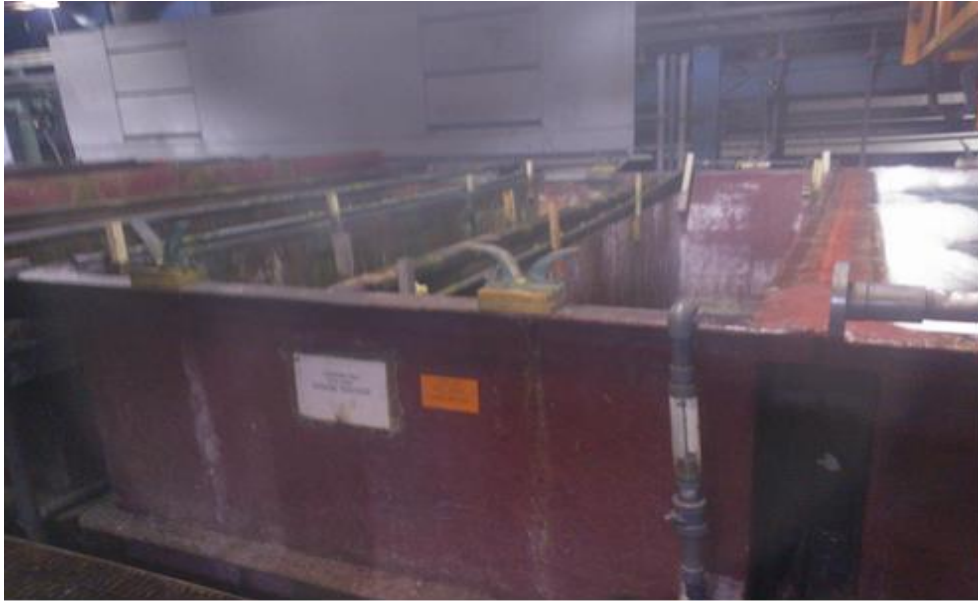
Exhibit 2. The chrome plating tanks.
