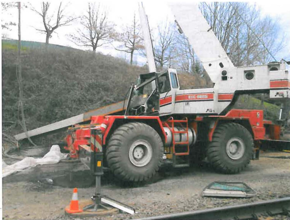
Figure1. Crane cab struck by H-beam.
