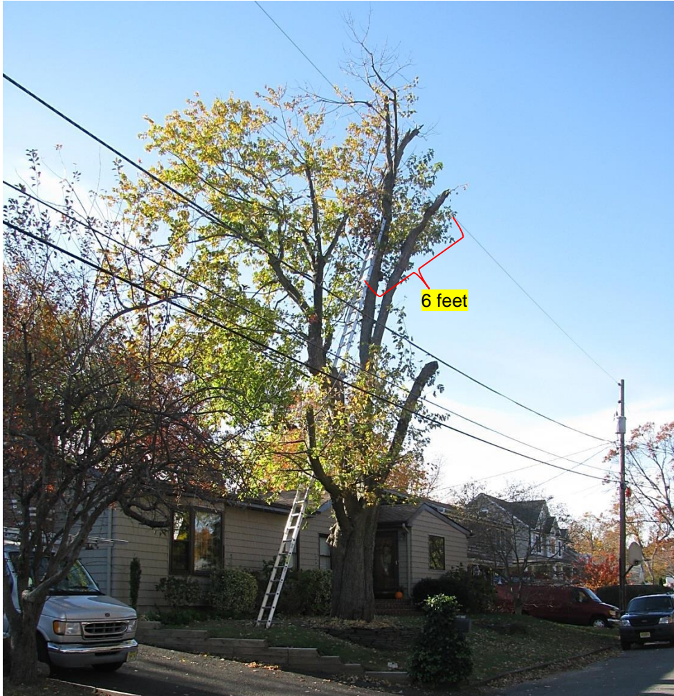
FIGURE 3. Branches to be cut near power line: a) full view; b) close up near wire.
