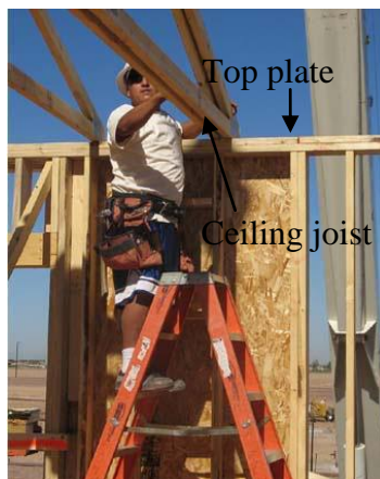
Figure 2 – Example of a construction worker setting a ceiling joist (connected to a roof rafter) on a top plate
