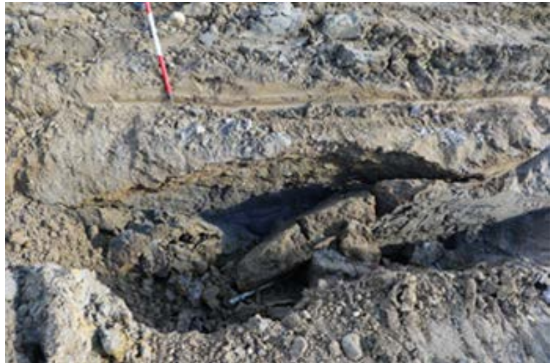
Figure 3. Trench wall collapse
