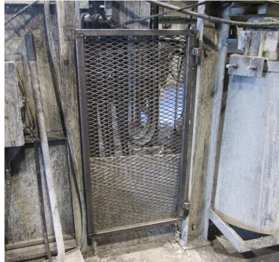
Photo 5. Installed guard with serpentine rubber strip visible (Photo courtesy of OR-OSHA).
