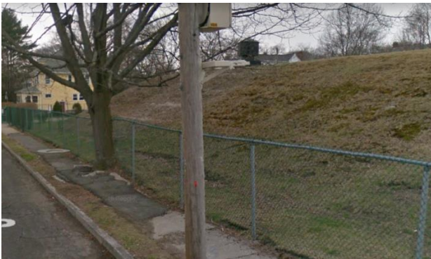
Figure 3 - One of the buckled sidewalk sections
