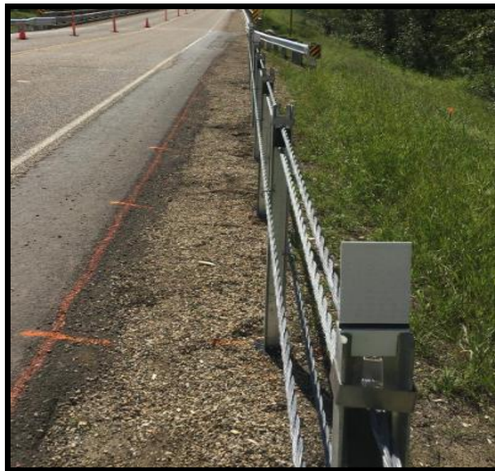
Photo 7. Cable barrier on right shoulder of highway 7 .
