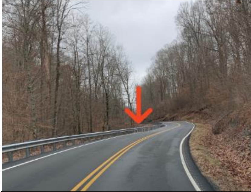
Photo 3. Photo representing the point in which the rear driver's side trailer struck and punctured the W-beam guardrail. Photo by and property of KY FACE.
