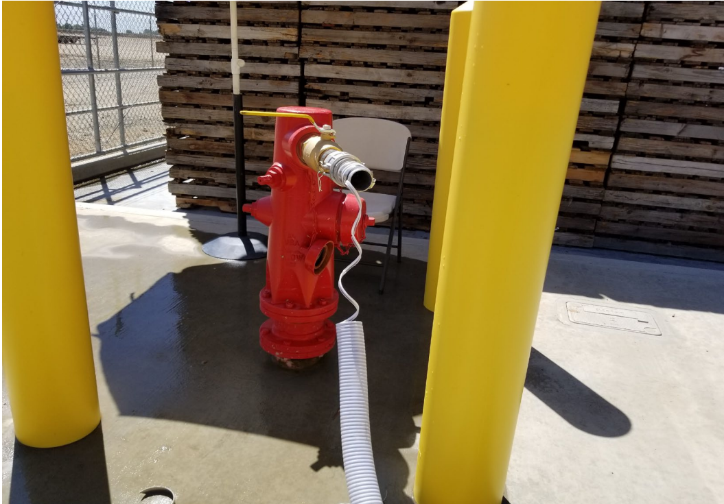
Exhibit 1. The fire hydrant involved in the incident.
