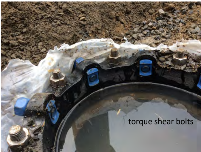
Photo 4. Flange bolts (silver) and torque shear (blue) on gland. Vertical riser has been removed. Note hex-heads of torque shear bolts are still attached. (Photo courtesy of OR-OSHA.)
