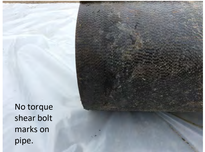
Photo 5. Bottom end of south vertical riser. Note there are no torque shear bolt marks on the outside of the pipe, indicating torque shear bolts were not tightened. (Photo courtesy of OR-OSHA.)
