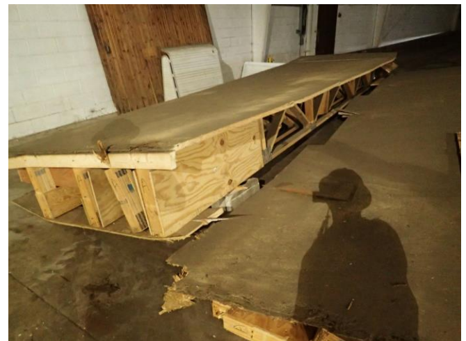
Photo 2. Example of truss/floor joists with foam-covered plywood that had previously been removed.
