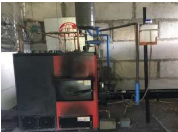
Figure 1 - The boiler/furnace and the auger/conveyor
