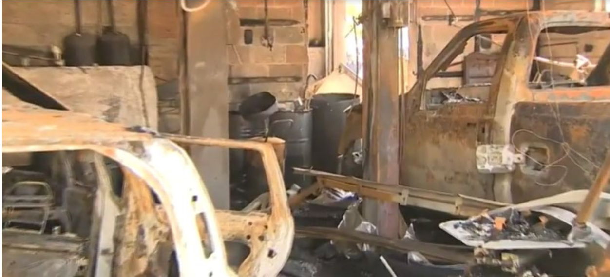
Figure 6 – Garage after the fire was extinguished, from scene footage; drums along back wall are in the center of the picture.
