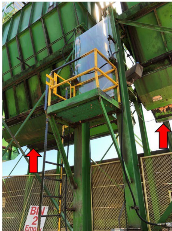
Photo 9: Bin control platform with ladder that truck drivers used to access hydraulic levers for bottom gates that released woodchips into the trailer. Arrows point to the gates.
