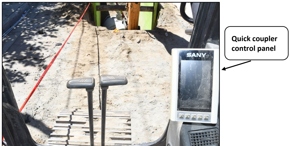
Exhibit 4. The control panel used to operate the quick disconnect. Photo courtesy of police department.
