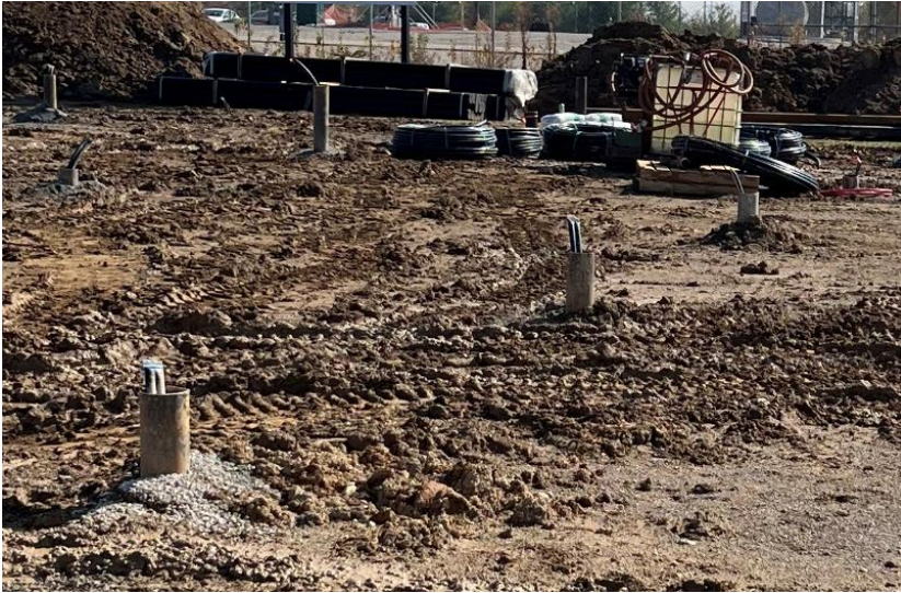
Photo 1. Geothermal system pipes (Property of KY FACE)
