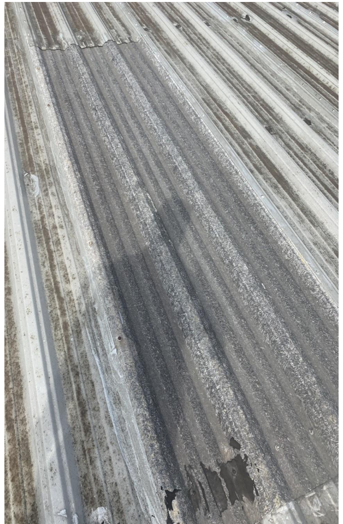
Photo 2. Photo showing 1 of 30 fiberglass skylights present on top of the building where the incident occurred (photo taken prior to incident).
