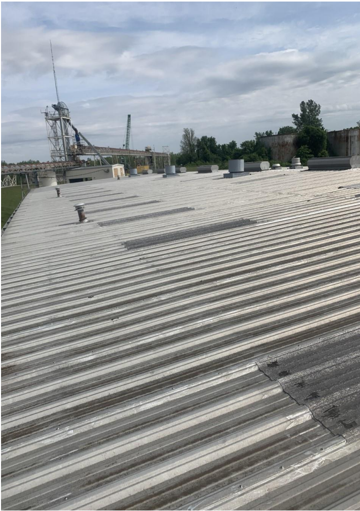
Photo 3. Photo showing fiberglass skylight arrangement and roof of the building where the incident occurred (photo taken prior to incident).
