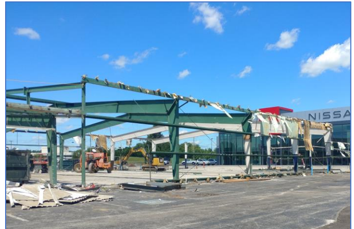
Photo 4. Building framework remaining at time of FACE site visit (Property of FACE program)
