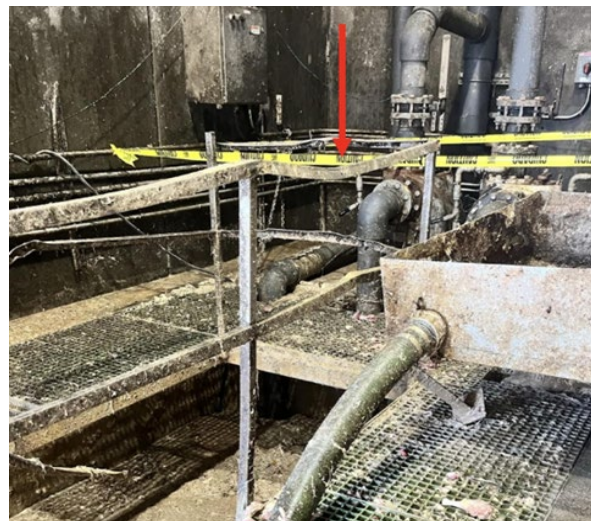
Exhibit 2. One of the damaged guardrails (red arrow) surrounding the offal pit. Photo courtesy of the employer.
