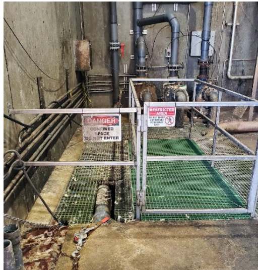
Exhibit 4. The new guardrails and floor grates that were installed after the incident. Photo courtesy of the CA/FACE program.
