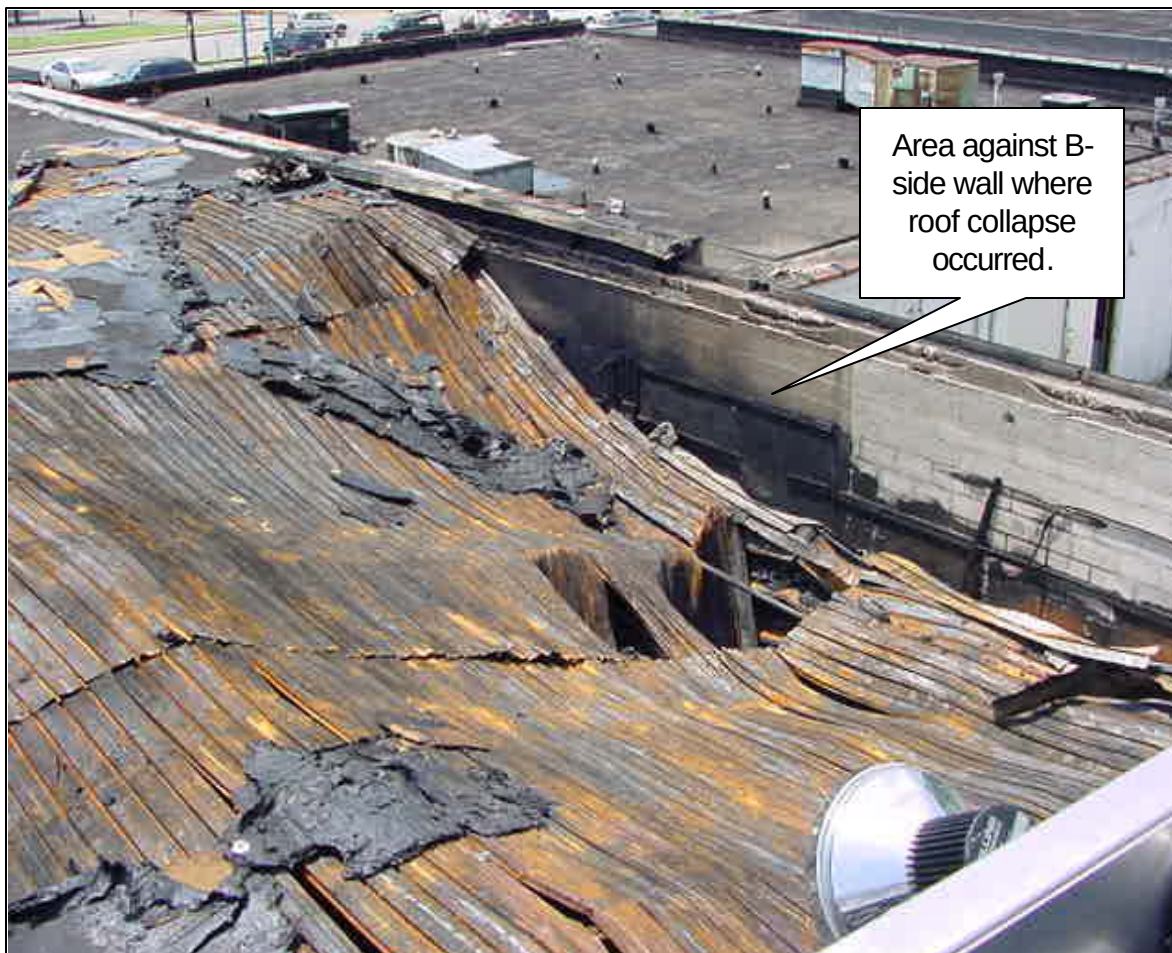
Photo 2. Roof collapse B-Side
