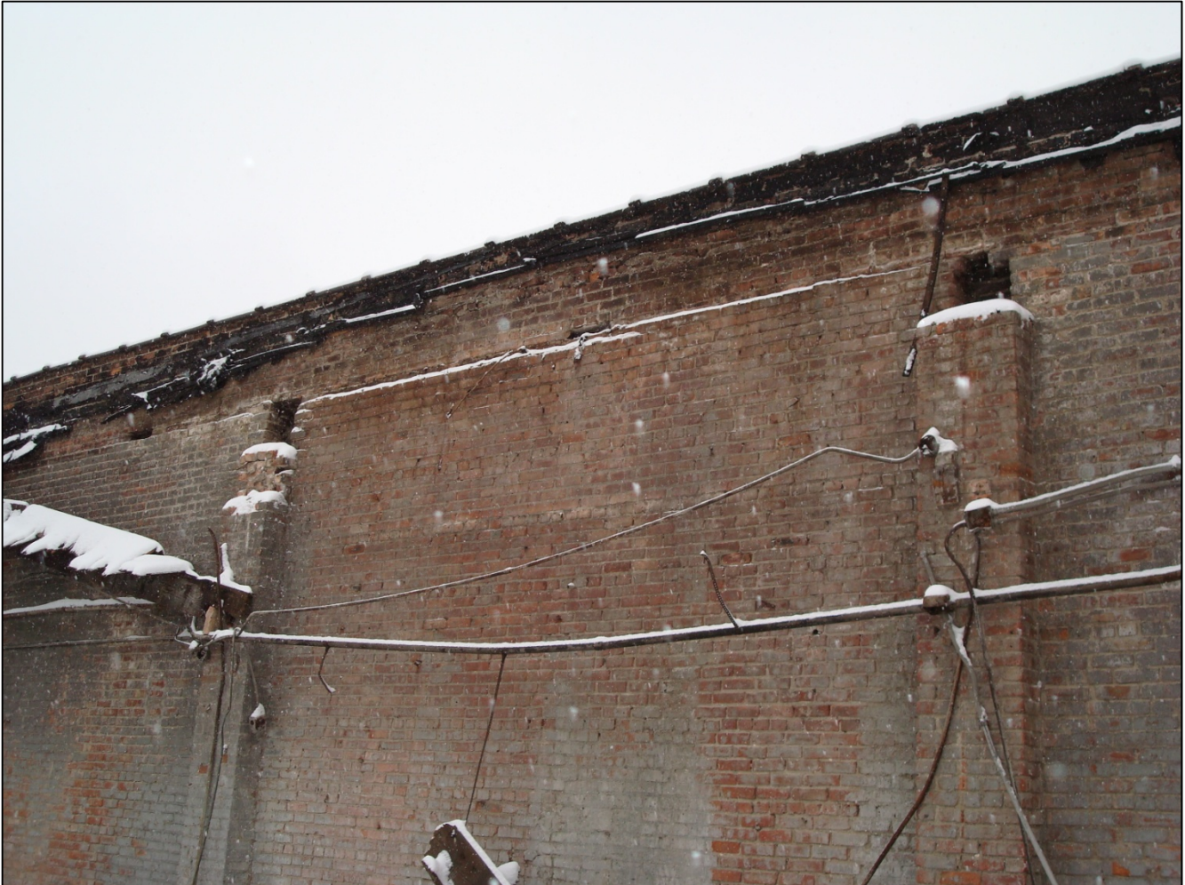
Photo 3. Photo shows the truss support pilasters built into the Sector 2 (west) wall. The Sector 4 (east) load bearing wall also contained support pilasters. The Sector 4 wall partially collapsed during the incident and was demolished after the recovery operations.
