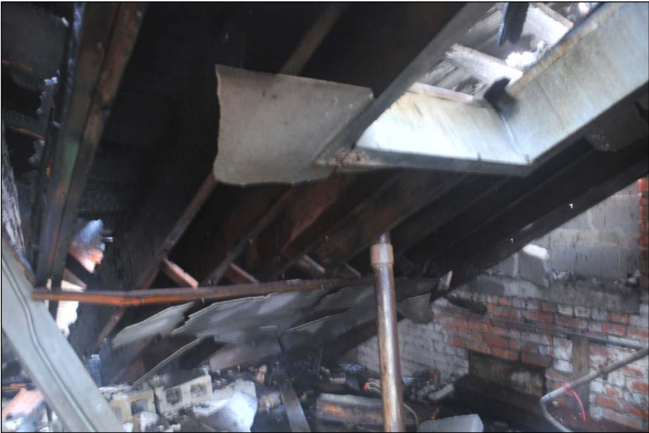
Photo 10. Photo shows the scuttle hole in the roof where the E-126 lieutenant looked into truss void for fire extension. Note condition of roof rafters indicates little fire damage in this area. (Photo courtesy of fire department)
