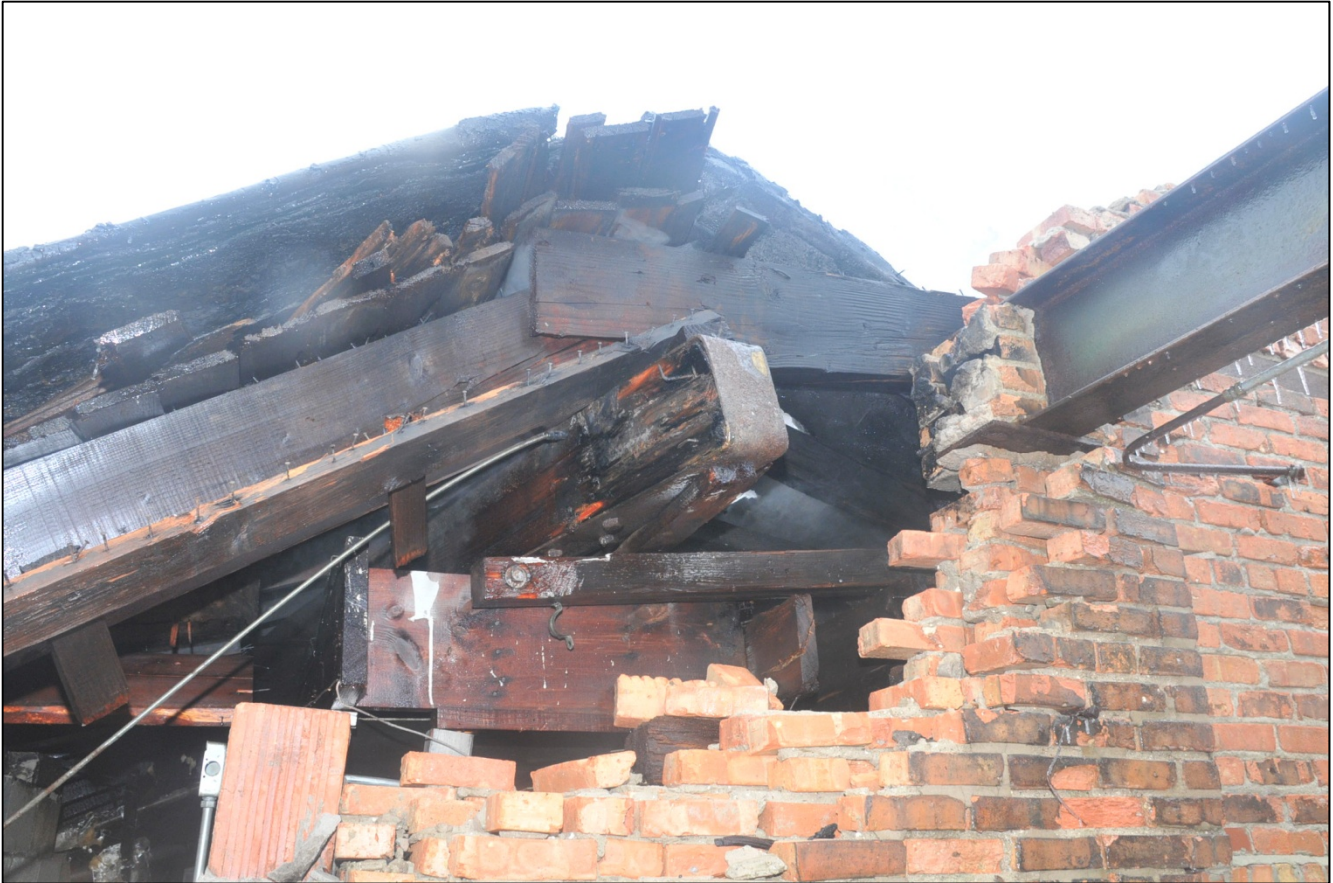
Photo 12. One end of heavy timber roof truss can be seen in center of photo. The truss has rolled over onto its side with the end penetrating through the Sector 4 wall. Photo was taken from the court yard on the Sector 4 side (facing west). (Photo courtesy of Fire Department)
