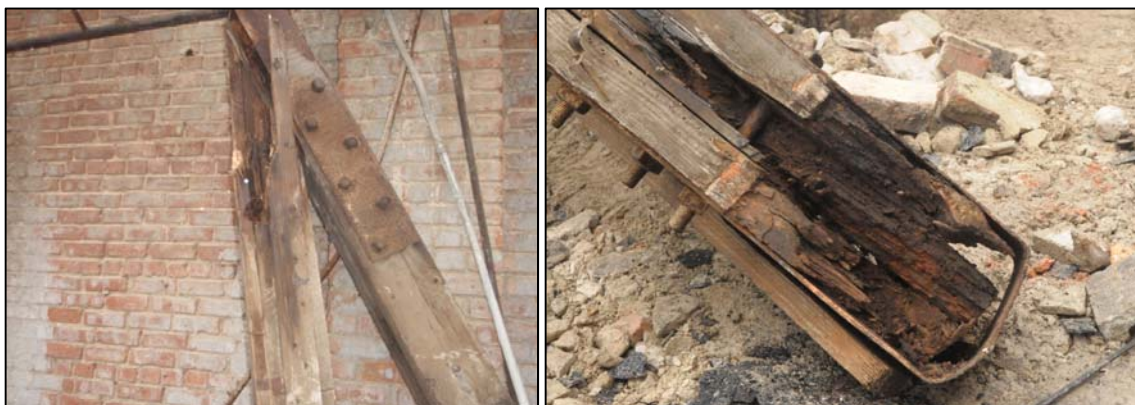
Photos show the deteriorated condition of bowstring roof trusses. Note the truss end in the left photo and the deteriorated condition caused by water damage in right photo. (Photos Courtesy of Fire Department Office of Fire Investigations)
