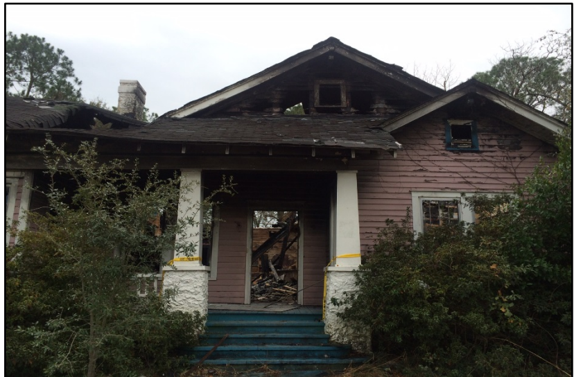
A lieutenant was killed during overhaul after a ceiling and roof assembly collapsed in this vacant building. (Photo by NIOSH.)
