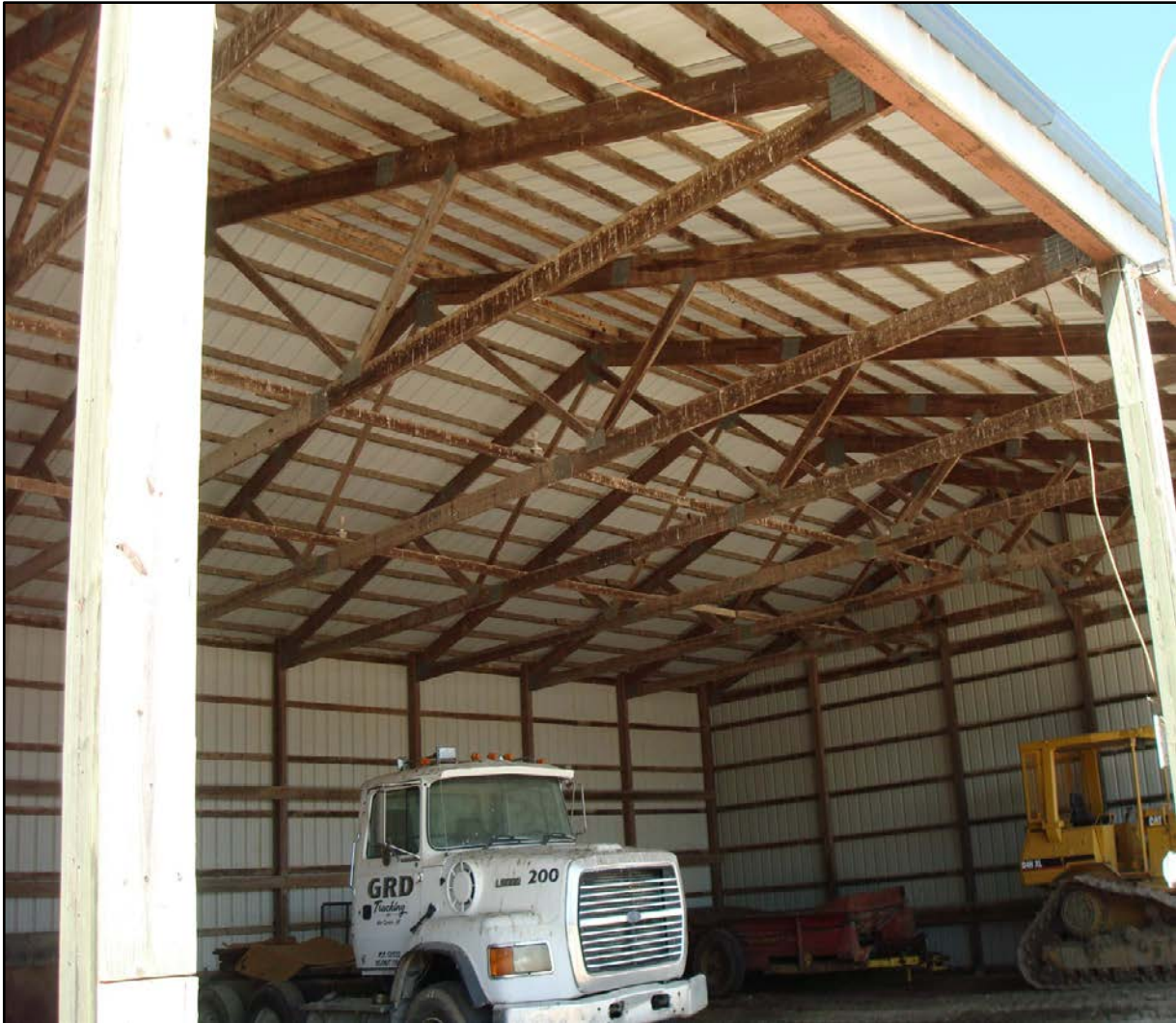
Photo 2. Similar building and roof construction on the property. This is an example of a pole barn without a pan ceiling, which the fire building had. A ceiling enclosure may leave the void area wide open from end to end.
