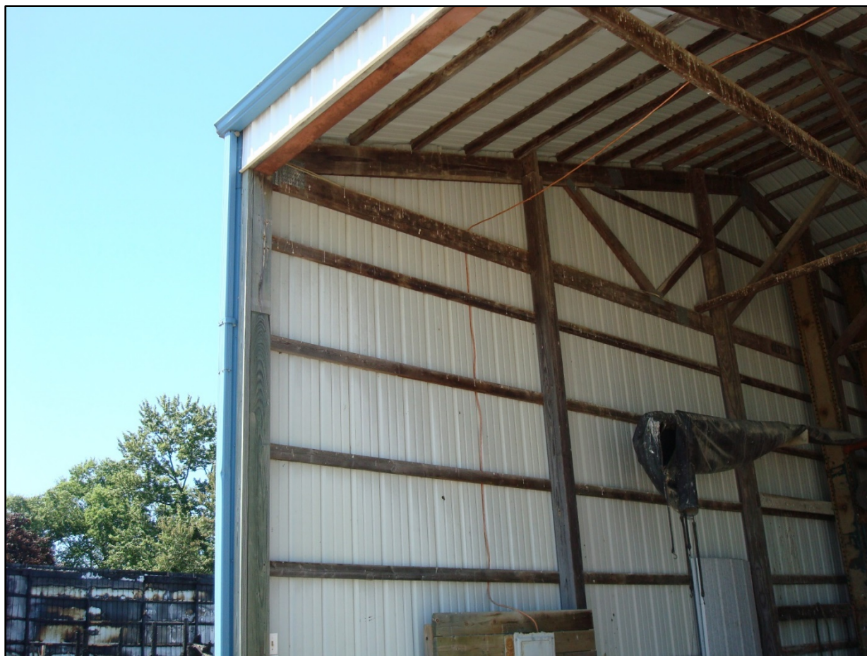
Photo 3. Similar building and roof construction on the property. Note the wide spacing of trusses. (NIOSH photo.)
