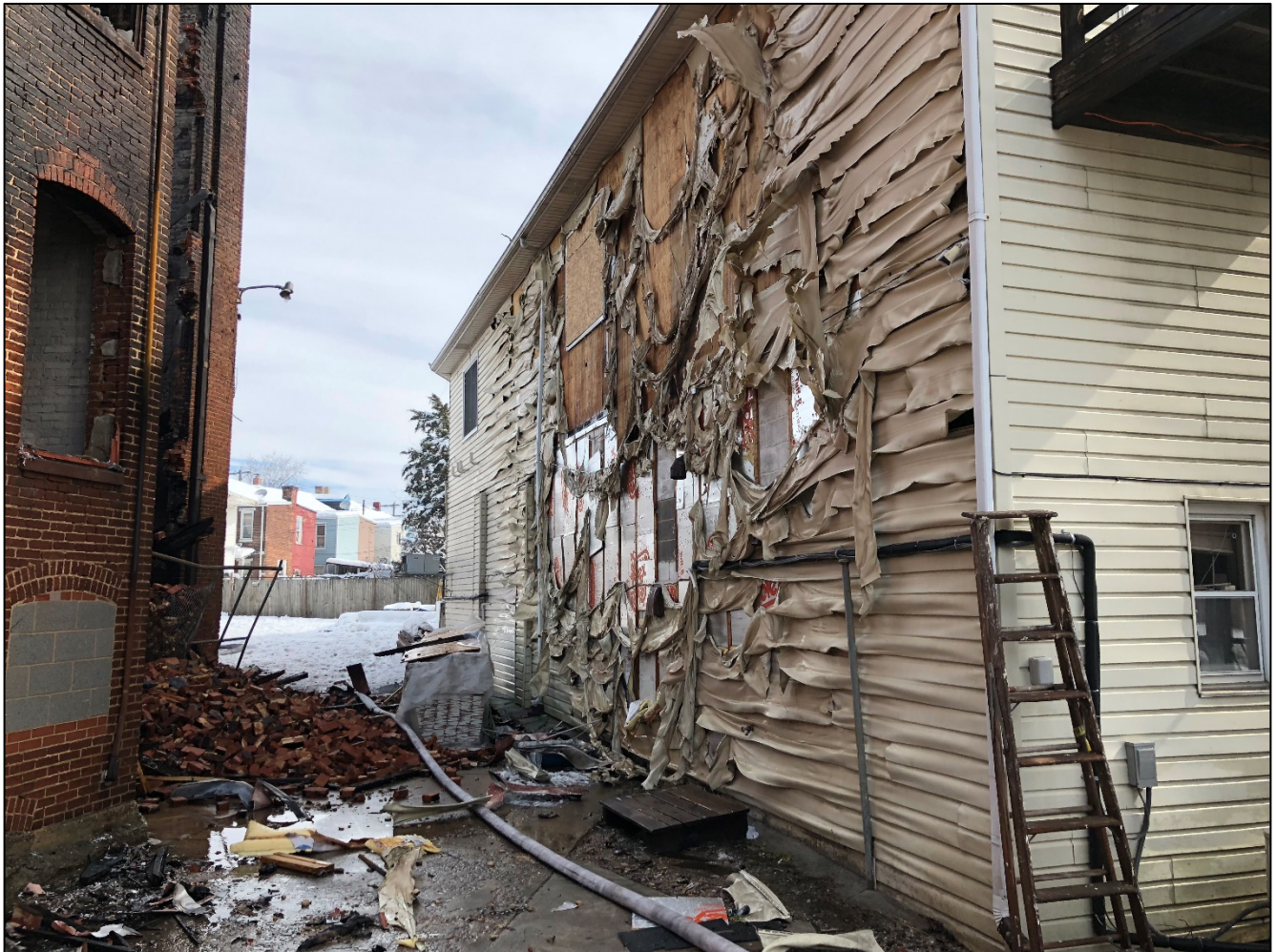
Photo 5. Photo shows heat damage to the rear of the building containing the beer distributor near the Side Delta / Charlie corner. (Photo courtesy of the Fire Department.)
