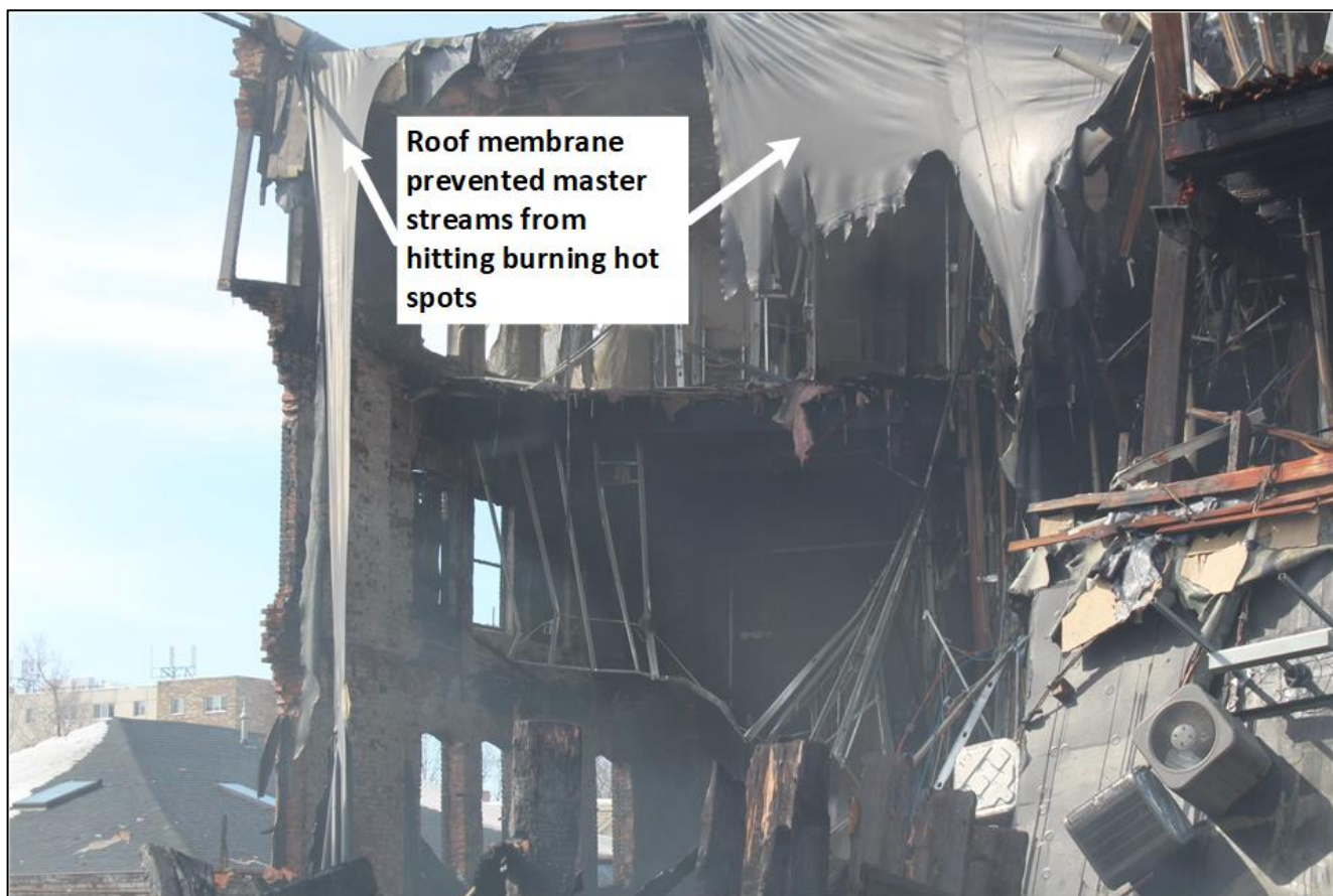
Photo 11. View from Side Charlie facing rear of remaining structure. Photo shows the partially melted roof membrane which deflected master streams and prevented water from reaching burning hot spots in roof and ceiling areas on the Division Three and Division Four. The inability to extinguish the burning hot spots ultimately led to the decision to enter the third and fourth floors to attempt to extinguish the remaining hot spots.
