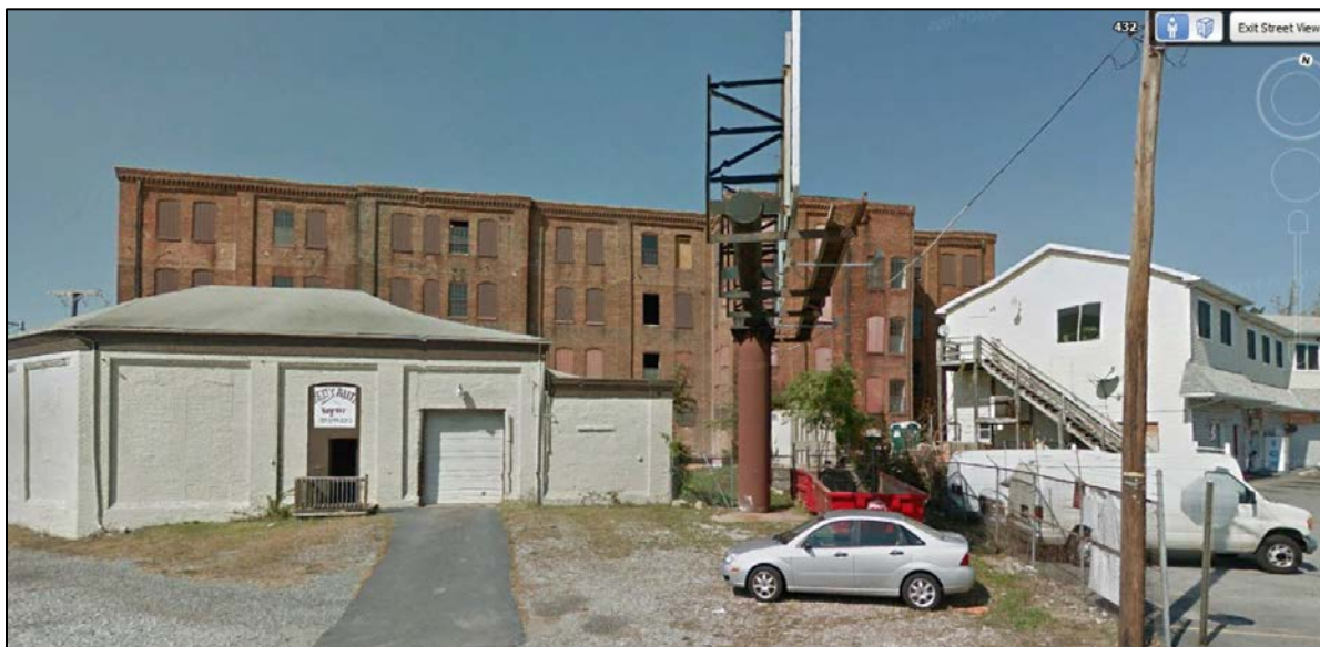
Photo 4. View of structure as seen from Side Delta facing north. (Photo adapted from Google Earth street view.)
