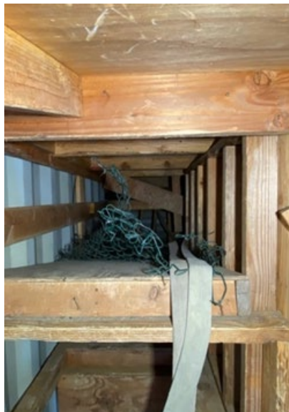
Figure 6. Diminished clearance. Photo by NIOSH.
