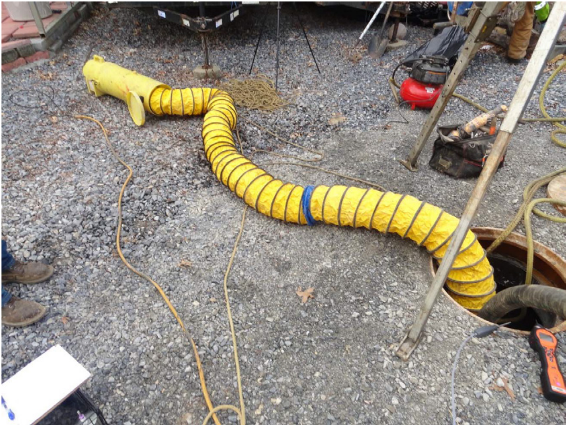
Figure 2. Manhole ventilation blower used to provide dilution ventilation to manhole during CIPP installation tasks, February 6, 2018.
