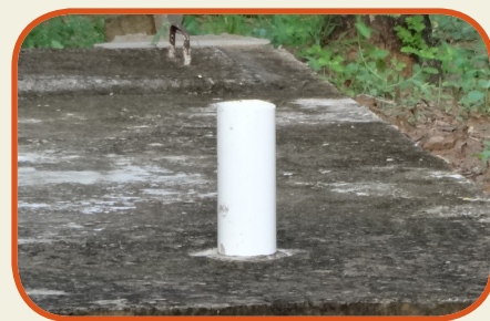
Cover ventilation pipes
