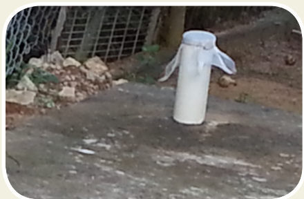
Septic tank ventilation pipe with screen mesh
