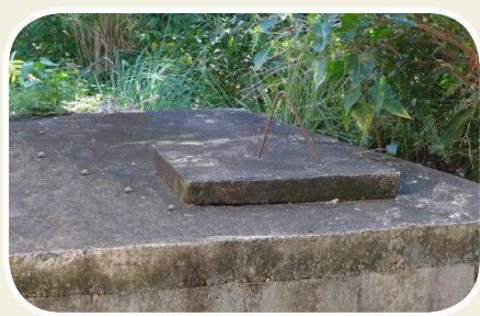
Septic tank with concrete cover
