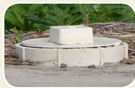
Septic tank sealed with PVC cap
