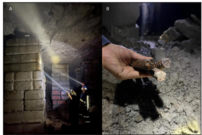
Figure 6. A) Photo of shear failure in roof and B) Photo of sheared bolts
