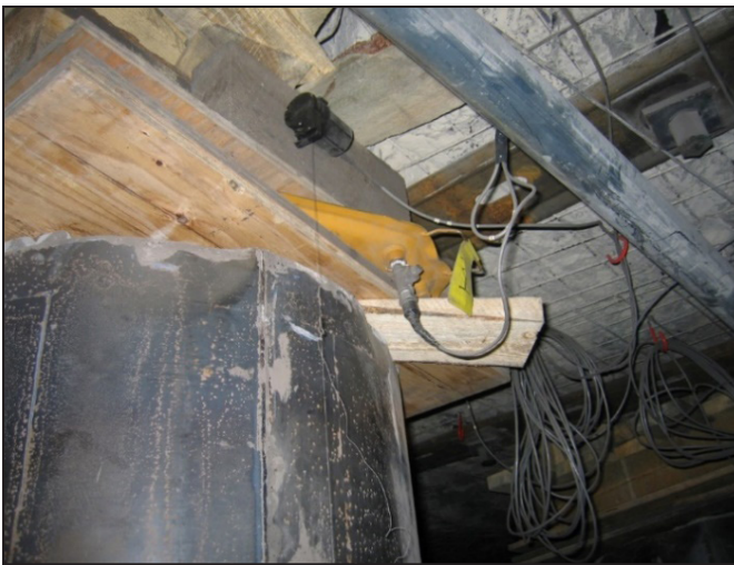
Figure 3. Complete extensometer installed on a can-type support in conjunction with a standing support load cell
