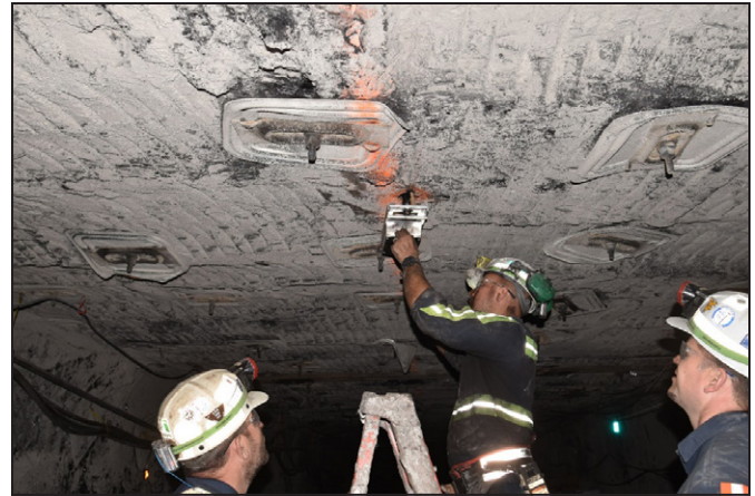
Figure 6. Installation of a multipoint roof extensometer depicting the insertion of mounting pipe into the borehole and securing with wedges
