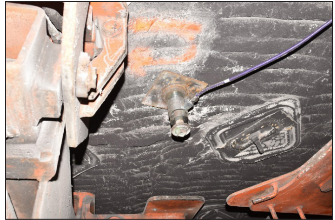
Figure 16. Completed installation of load cell on a cable bolt using the NIOSH installation procedure
