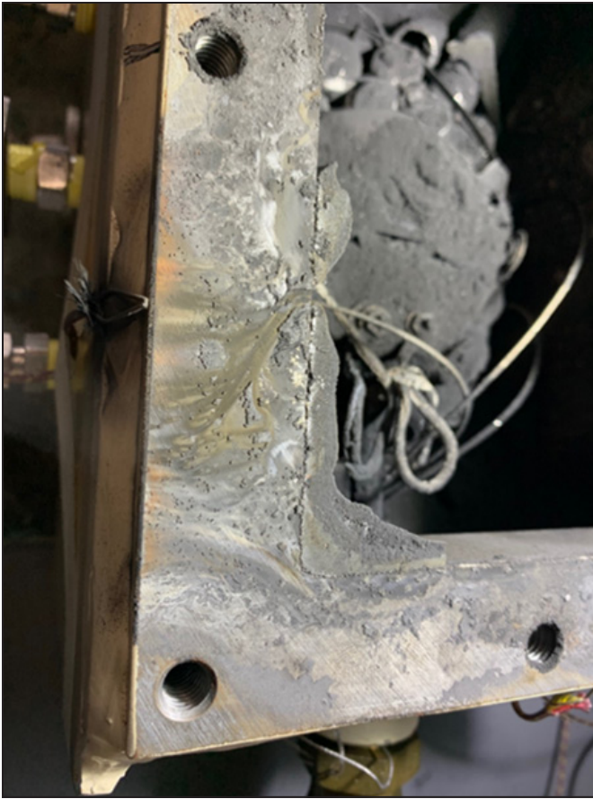
Figure 11. Escaping gasses etched a path through soot that accumulated in the cover joint
