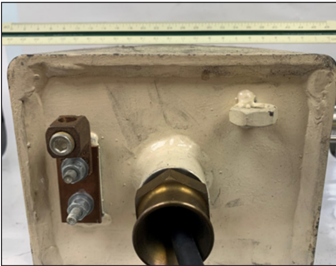
Figure 12. Thermal runaway pressure deformed the XP enclosure bottom plate beyond allowable limits
