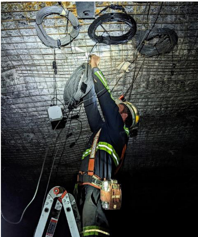
Figure 15. Example of a researcher safely using a ladder to hang cable from the mine roof.
