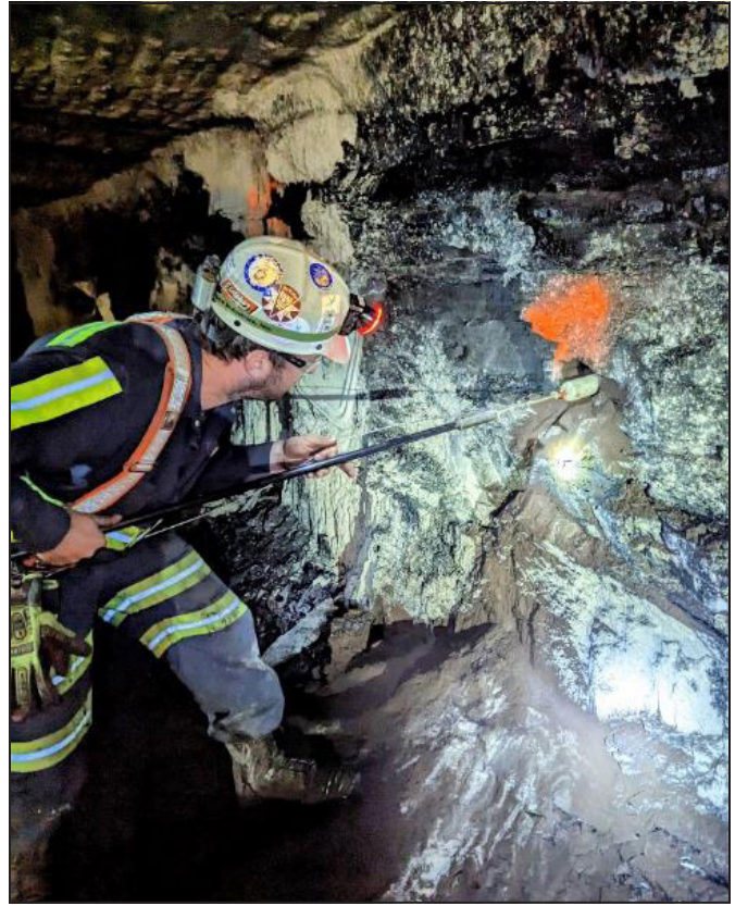
Figure 7. Photo depicting a researcher beginning the installation of a BPC using a set of insertion/setting rods
