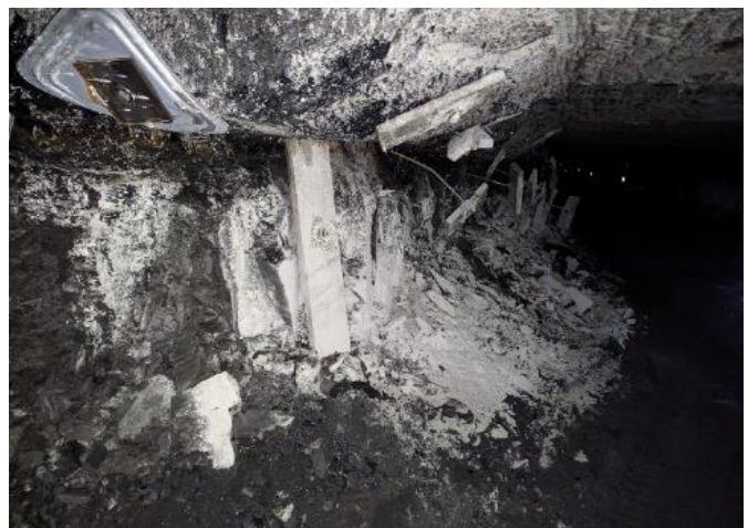
Figure 19. Example of rib sloughage, loose rib bolts, and the potential for brow formation of a coal rib
