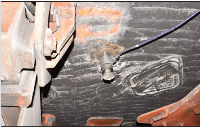
Figure 13. Example of an installed roof bolt load cell
