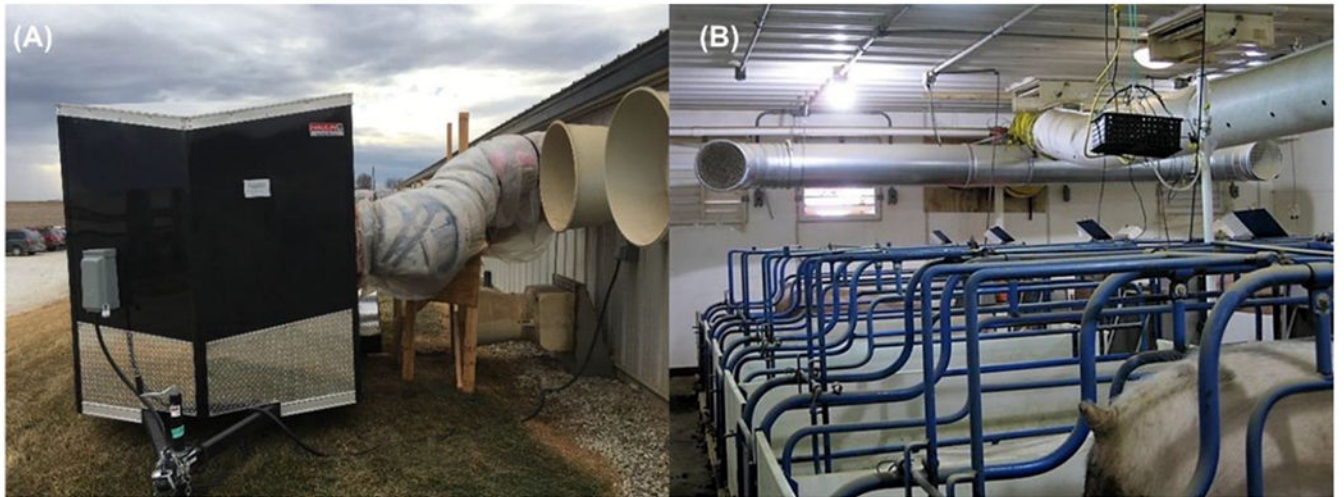
Figure 2. Ductwork installed in the treatment room: (A) outside attached to air handling unit and (B) inside the treatment room.
