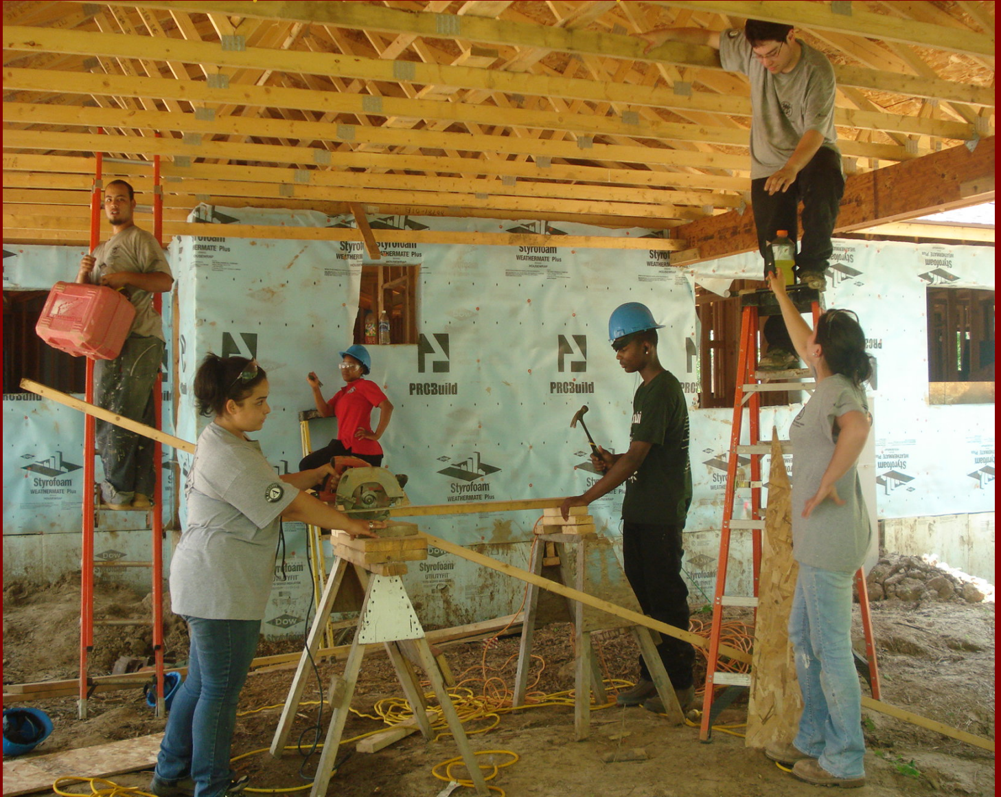
1. Untidy housekeeping 2. Cord in puddle of water 3. Facing outward on ladder 4. No 3-point contact on ladder 5. Improper use of step ladder 6. Missing 4 to 1 ratio on extension ladder 7. Standing on top rung 8. No hand hats 9. No safety glasses 10. Ring on finger 11. Incorrect use of hammer 12. Incorrect hand placement when using tools 13. Hammer placed on top of ladder 14. Incorrect passage of open utility knife 15. Inattentiveness when using power tool 16. Headphones
