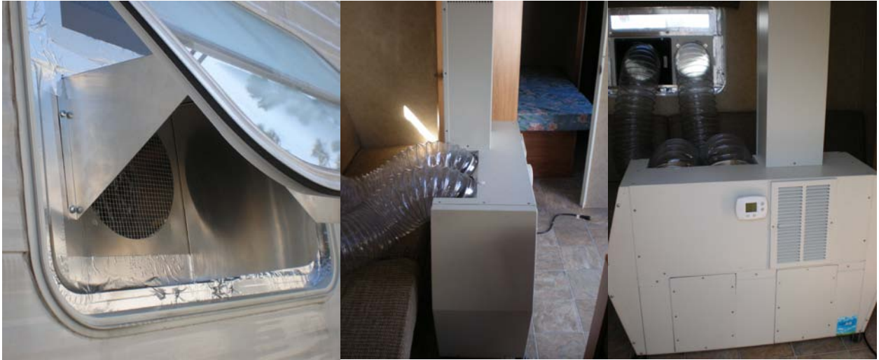
Figure B-5. HEPAiRx unit placed in Trailer 5.
