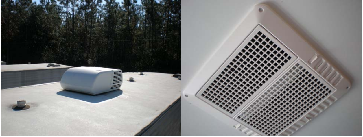
Figure B-17. AirXcel unit installed in Trailer 15.
