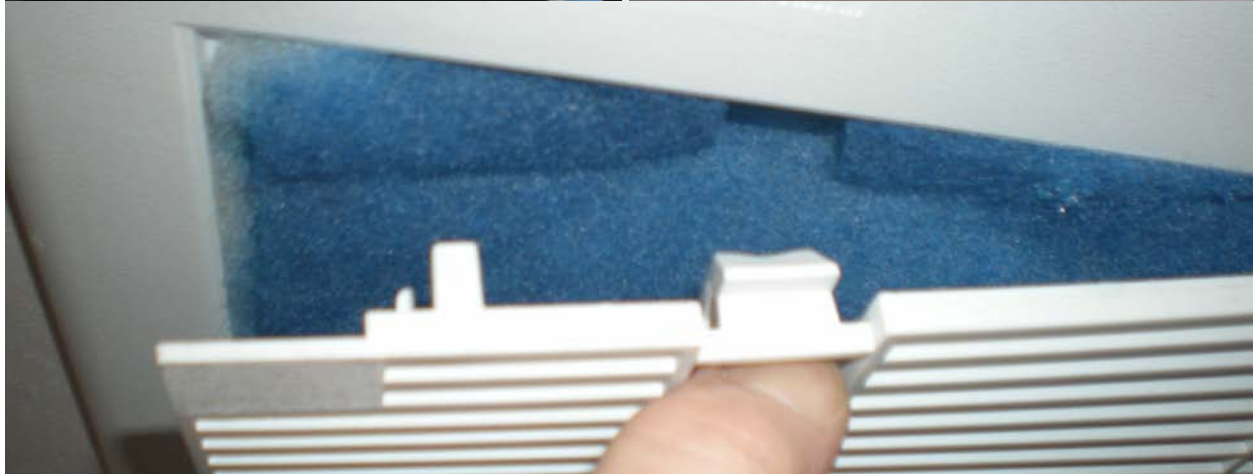
Figure B-1. Remov filters placed in Trailer 1.
