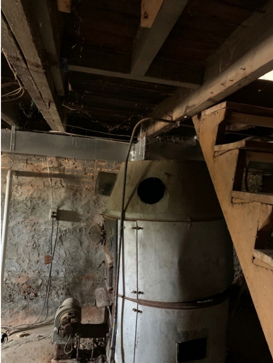
Photo 3: Furnace, Stairs to the Basement, and Basement Ceiling
