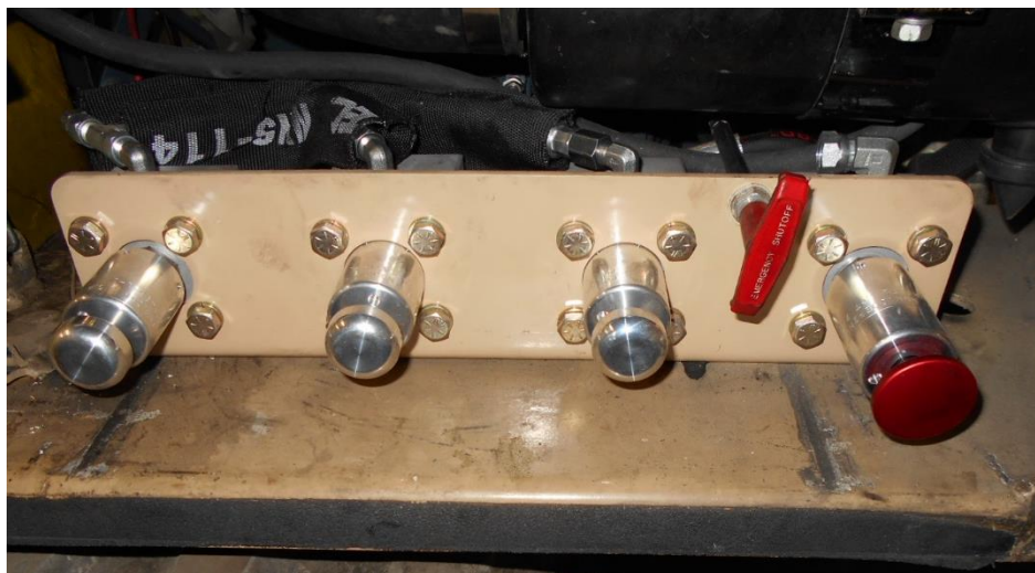
Figure 11 – Manual Control Valves
