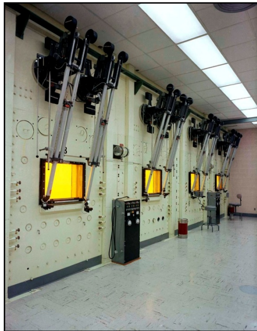
Fig. 8-2. CMR Building Wing 9 hot cells
