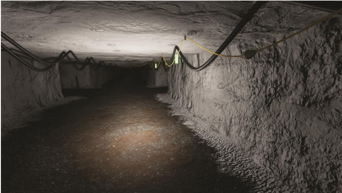
Figure 10. Screen captures from VR Mine depicting mine infrastructure that can be used in the KSA of wayfinding.
