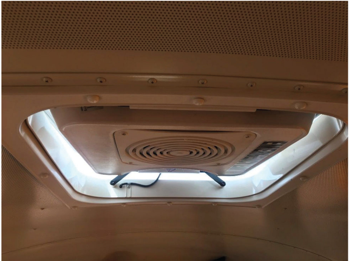
Figure 2. “Scooped” configuration of the ceiling hatch, with only the distant side of the hatch tilted upwards.
