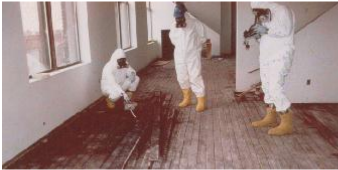
Workers in protective gear examine mercury under floorboards at residential building. Photo by Jim Pasquale, New Jersey Department of Health.
