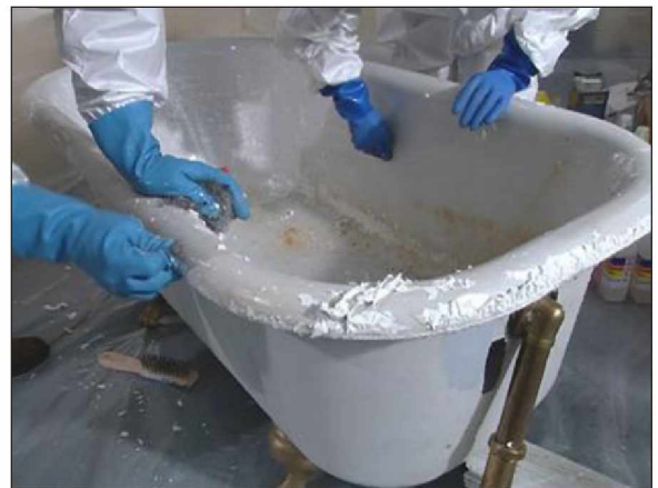
Workers use a methylene-based stripper to remove paint from a bathtub prior to refinishing.
