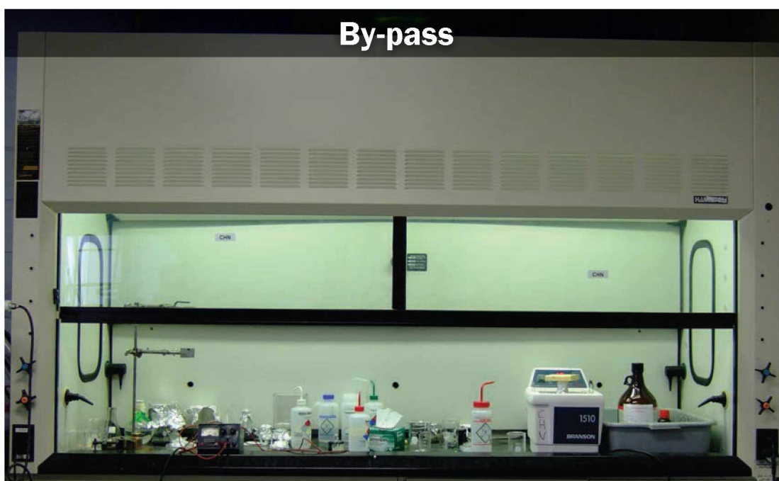
Figure 11. Laboratory bypass hood (note the by-pass chamber above the sash).
