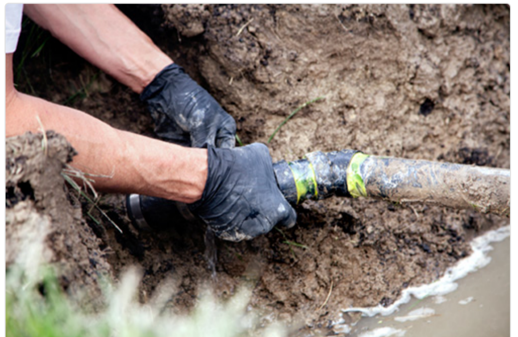
Water infrastructure requires regular maintenance.
