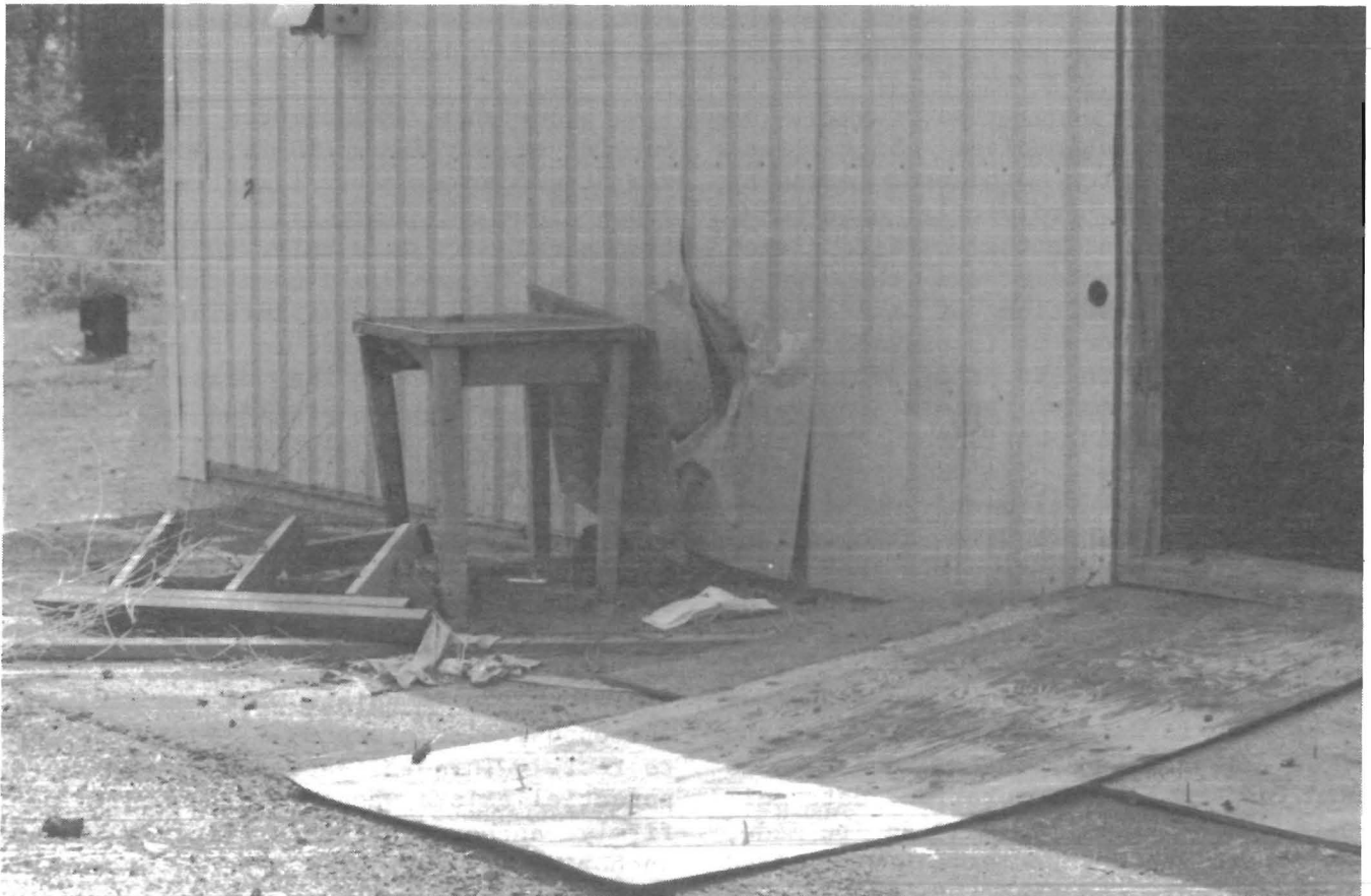
FIGURE 16. - Wall penetrated by projectile.
