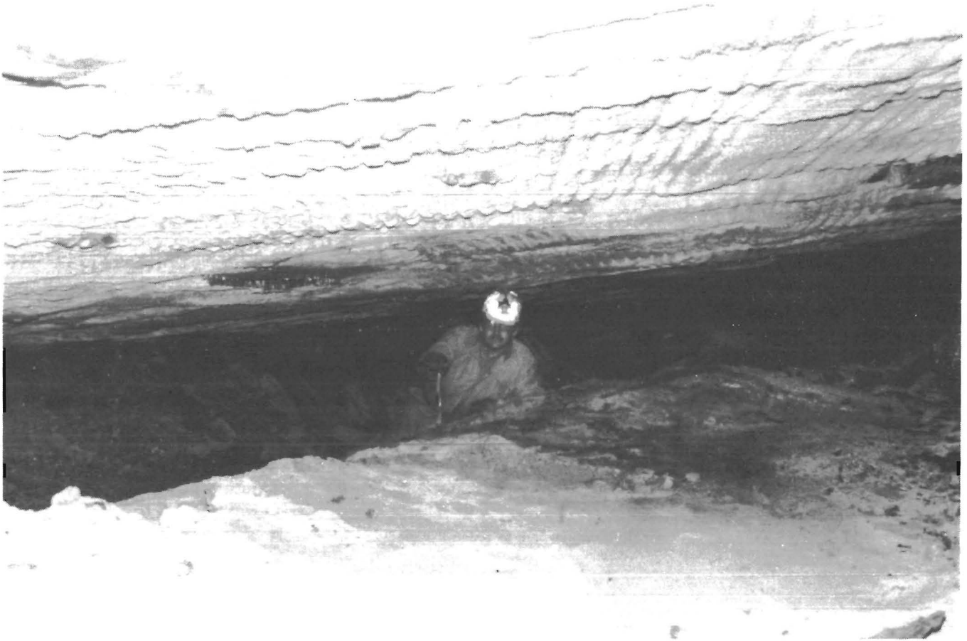
FIGURE 13.—Major floor heaving and rib spalling occurring in lower mine.
