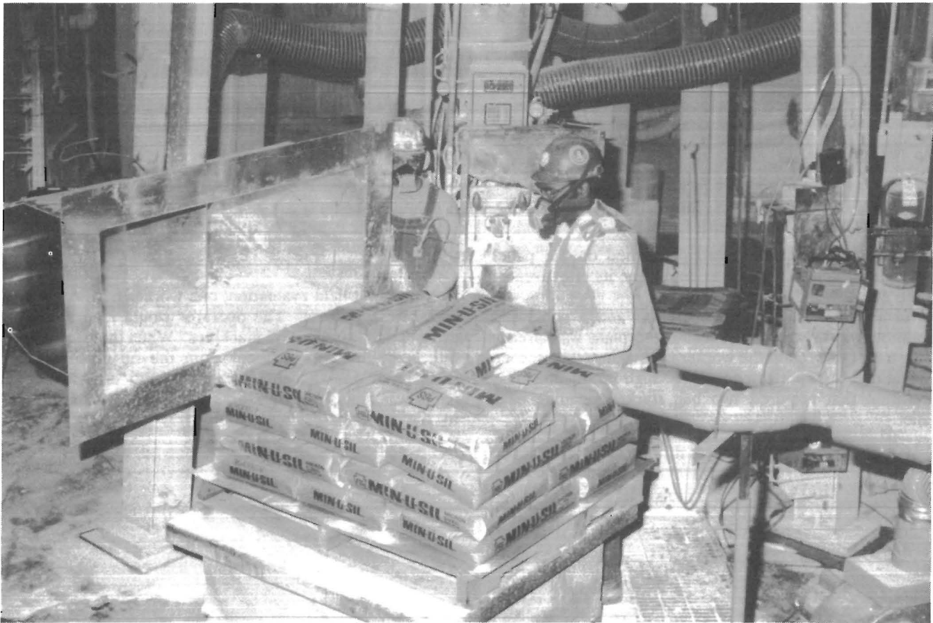
Figure 3.-Pallet loading dust control system at field site 1.
